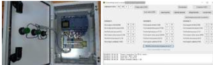
Figure. 17 Smart lighting automation add-on unit and configuration program
